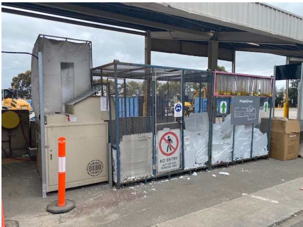
Total footprint area SH-150S and EPA cage approx. 6m (L) x 2m (W) x 3m (H)
