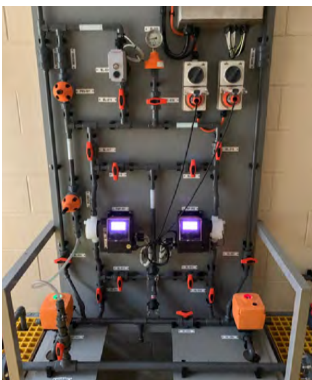
Bulgun - Chlorine dosing board and pump units.
