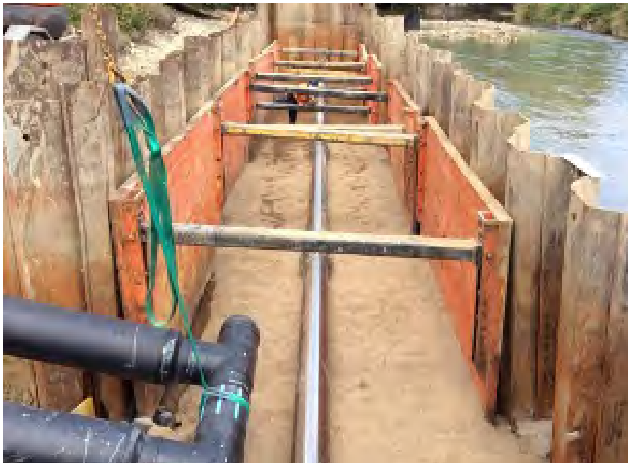
South Liverpool Creek Intake filter – S/S intake screen is 300mm dia 22m long. Bedded in sand surround 2.5 - 5mm grading.
