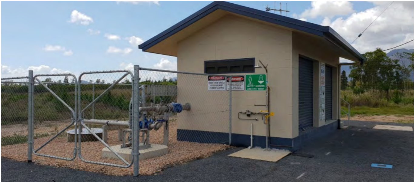
Kennedy Bore and Chlorine Dosing Building/Switchboard Enclosure.
