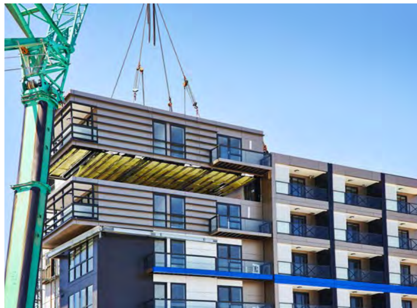
One9 apartment tower, Amnon Weber Architects (2014), Melbourne. Constructed in five days using the Hickory Group's UB® System. https://www.architectureanddesign.com.au/editorial/industry-news/nine-storey-melbourne-apartment-goes-up-in-just-fi
